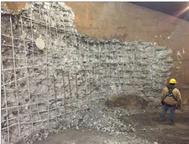
SLSDC crews working on demolition of deteriorated/damaged concrete for replacement by a contractor in the south filling and emptying culvert at Eisenhower Lock during the winter months of 2017.
