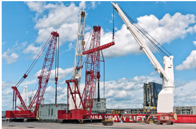
Offloading Transformers from one of the 4 HHL ships at the Duluth Port Authority.
