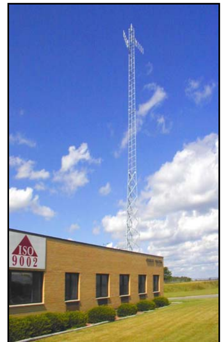
AIS Shore Base Station at Eisenhower Lock
