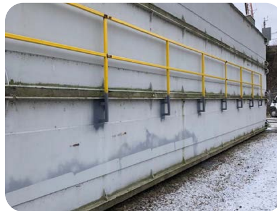
Fixed Guard Rail System
