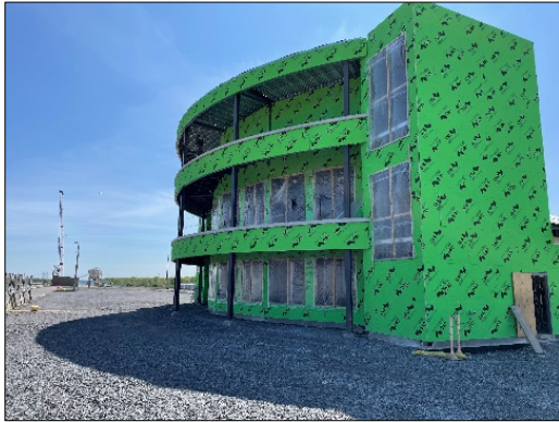
Construction of the new Seaway Visitor Center at Eisenhower Lock. Work is expected to be completed in late 2023.
