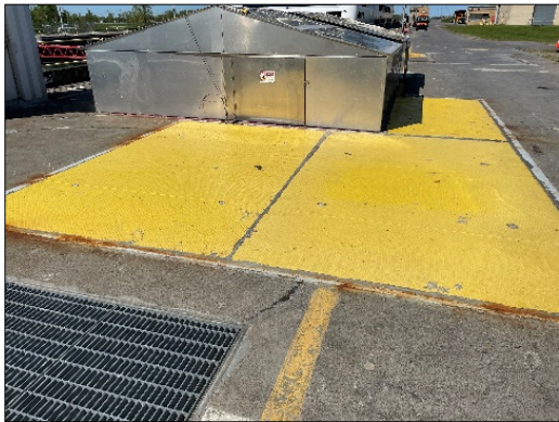
Completed culvert valve recess cover on the downstream north side of Snell Lock.
