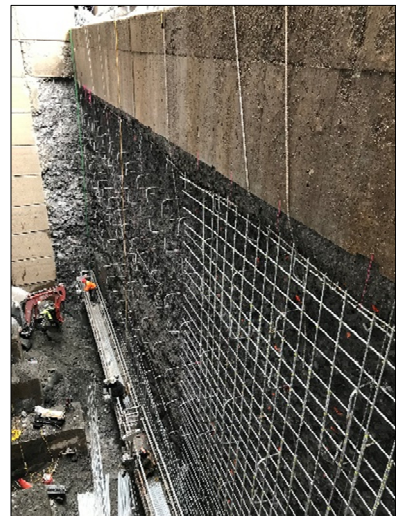
Contractors working on concrete replacement in the vertical lift gate at Eisenhower Lock in the winter of 2022.
