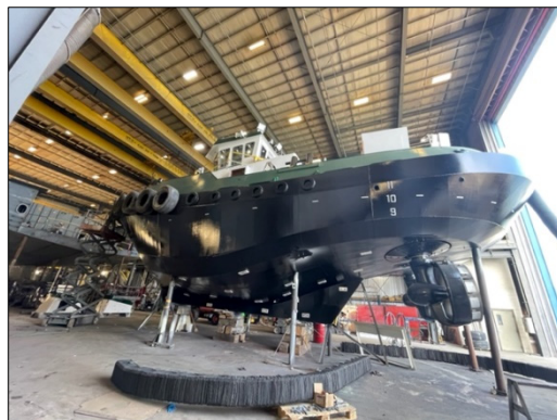
Construction of the GLS’s 60-foot SEAWAY TRIDENT tugboat at the Washburn & Doughty Shipyard in East Boothbay, Maine.
