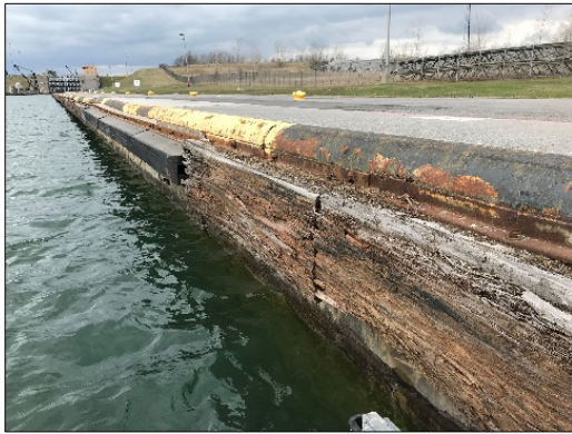
Section of ship fendering on the downstream side of Eisenhower Lock (old wood fendering on the right side of photo with newly installed rubber fendering on the upper left)
